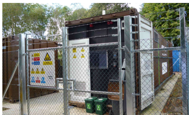
MUCKBUSTER® system at USSP Science Park
